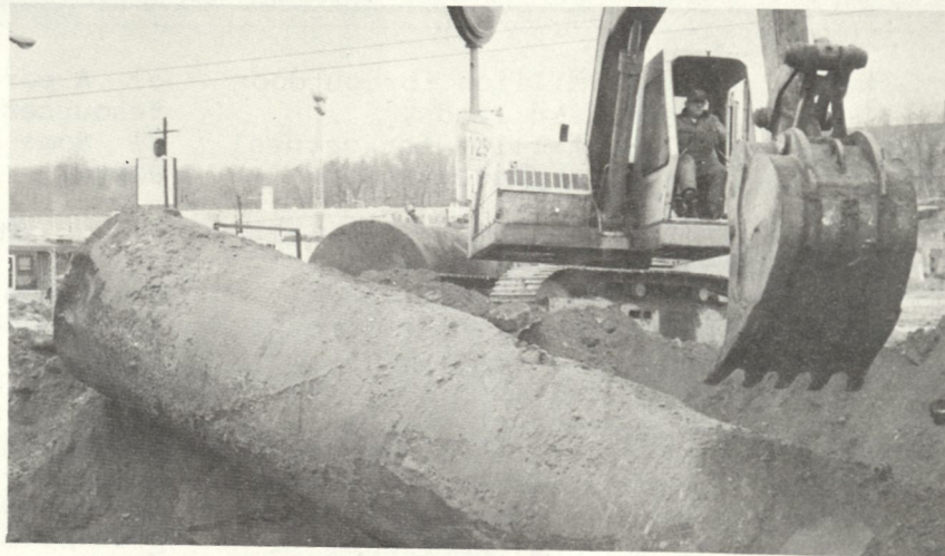
Underground storage tanks, installed in the 1950s, are being replaced to comply with new regulations to protect groundwater. (Photo: Robert Paier)
